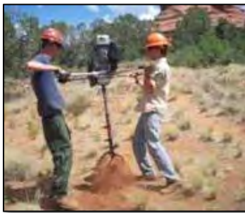
Trail coordinator, Paul Hart (left) works with a YCC member to drill fence post holes.
